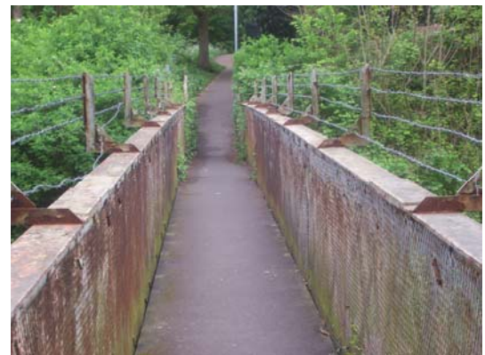
Restricted width across railway overbridge. “Cyclists please give way to pedestrians” signage required
