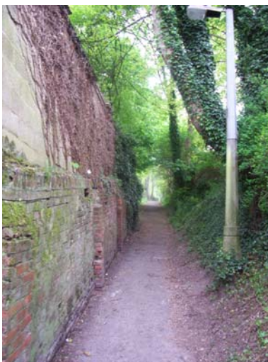
Narrow section at bottom section of Milford Hollow looking up hill towards railway overbridge – widening work required
